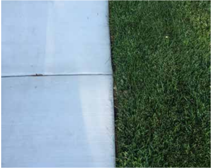
After Repaired sidewalk, high repetitive maintenance costs
