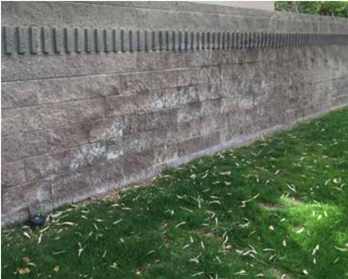
Wall damage from sprinklers
