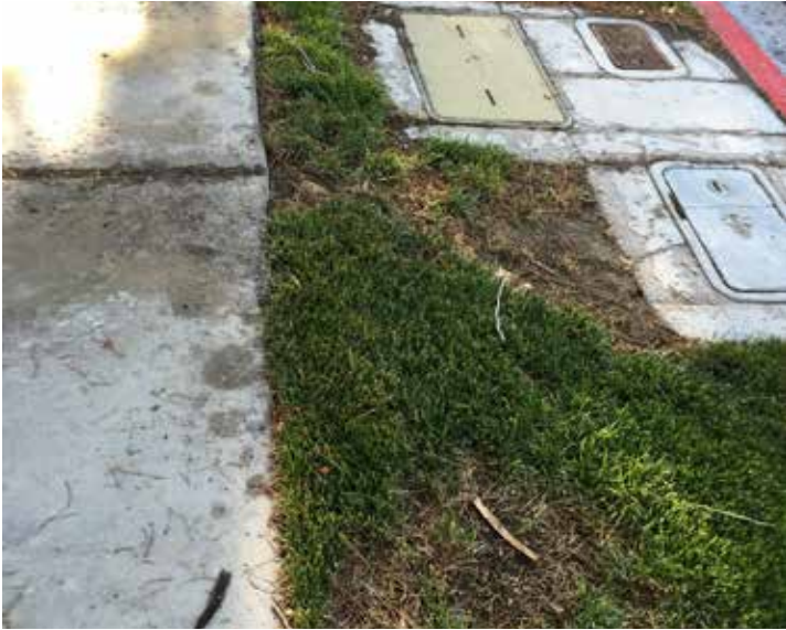
Before Sidewalk damage from overspray
